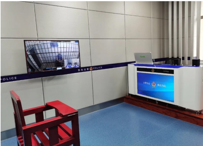
Tiandy interrogation system installed in Baotou Province, China, in 2020. Source: Tiandy.
